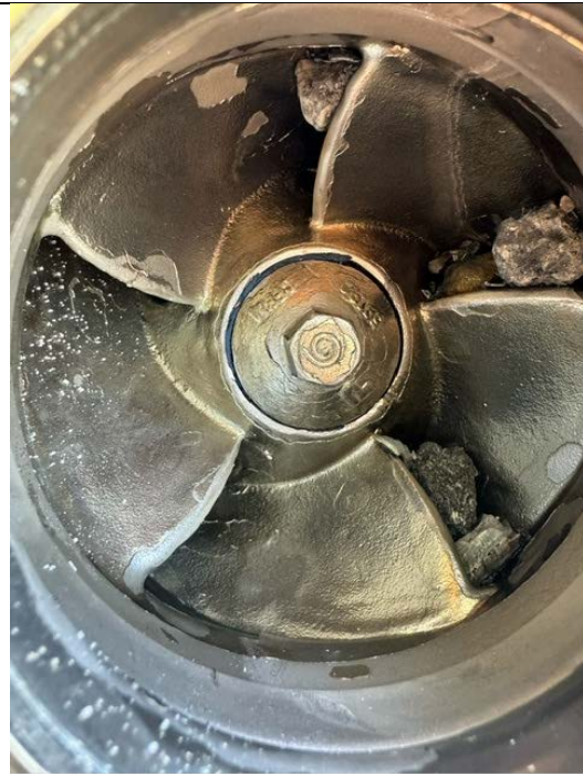
Pump impeller obstructed with large pieces well formation material.
