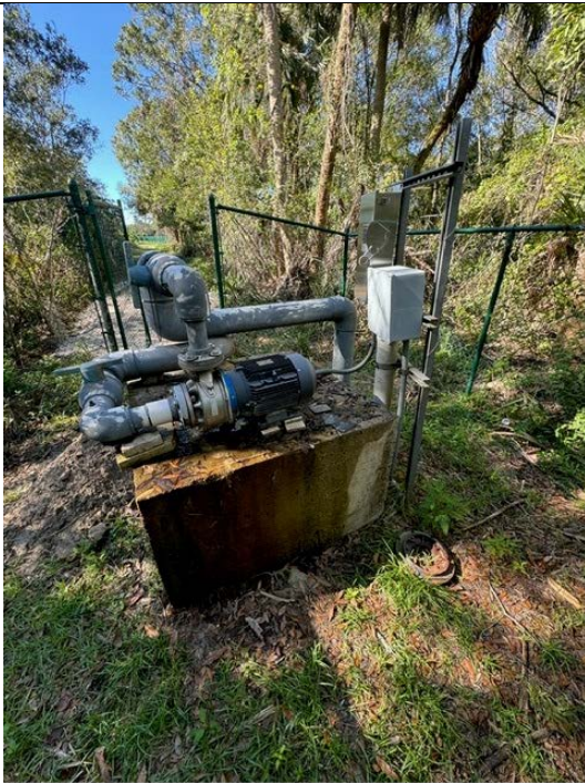
Well Pump - Site location.
