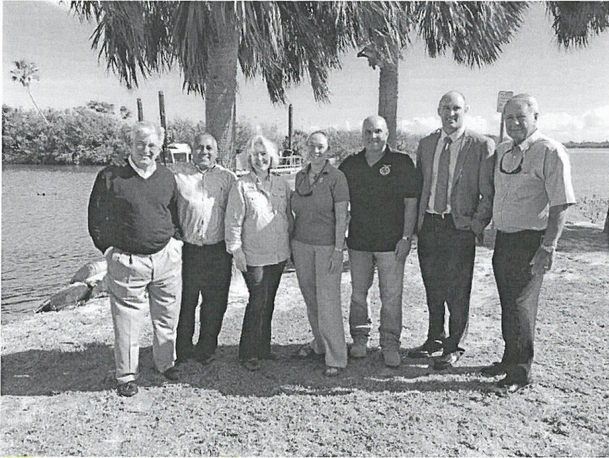
District Executive Director Dr. Ann Shortelle and partners gathered Nov. 30 to celebrate the Cocoa Beach dredging project.
