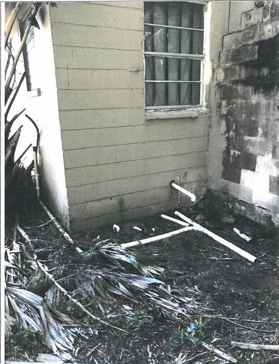
5/8/18 9:33am Photo 1A Discharge Pipes coming from Church(Structure A)
