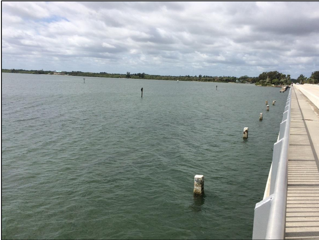
Damaged Wabasso Fishing Pier – East and West Structure – Photos taken April 13, 2017
