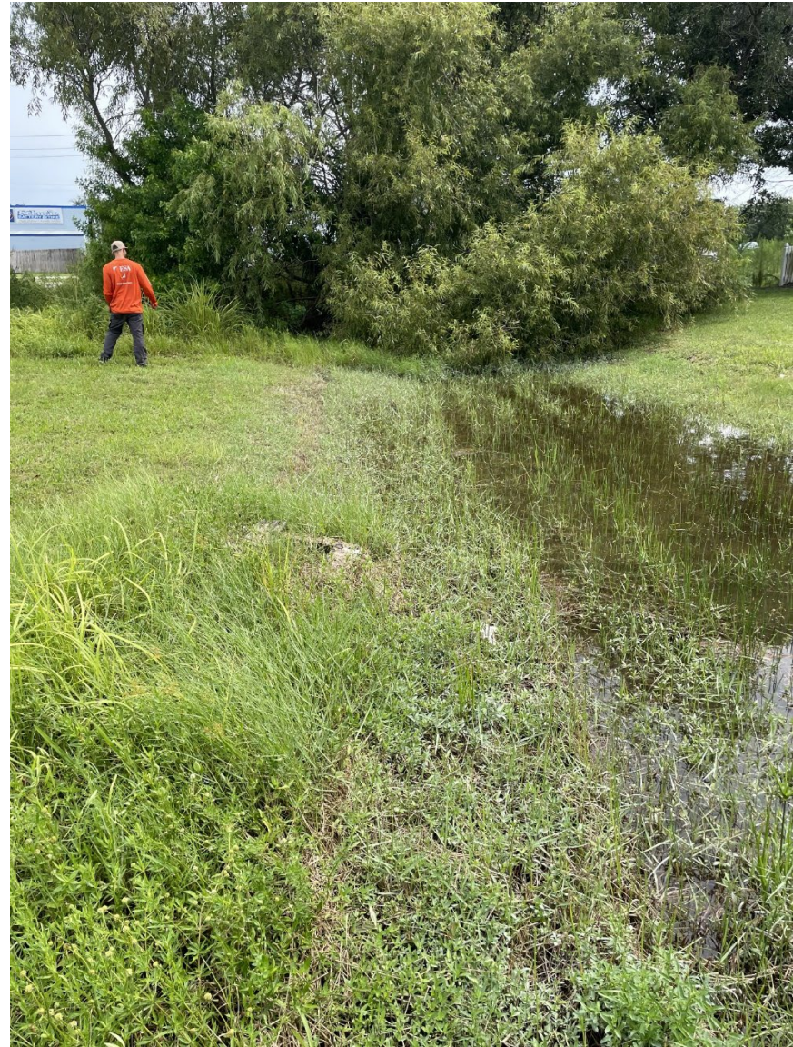
Figure 4. Swale full of water behind Inn, #2
