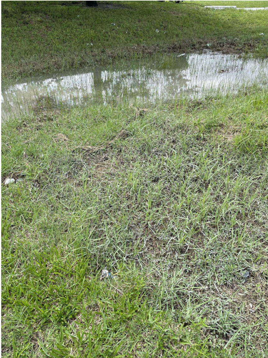
Figure 3. Swale full of water behind Inn, #1
