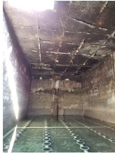
Figure 2 - Concrete spalling in the tank now.
